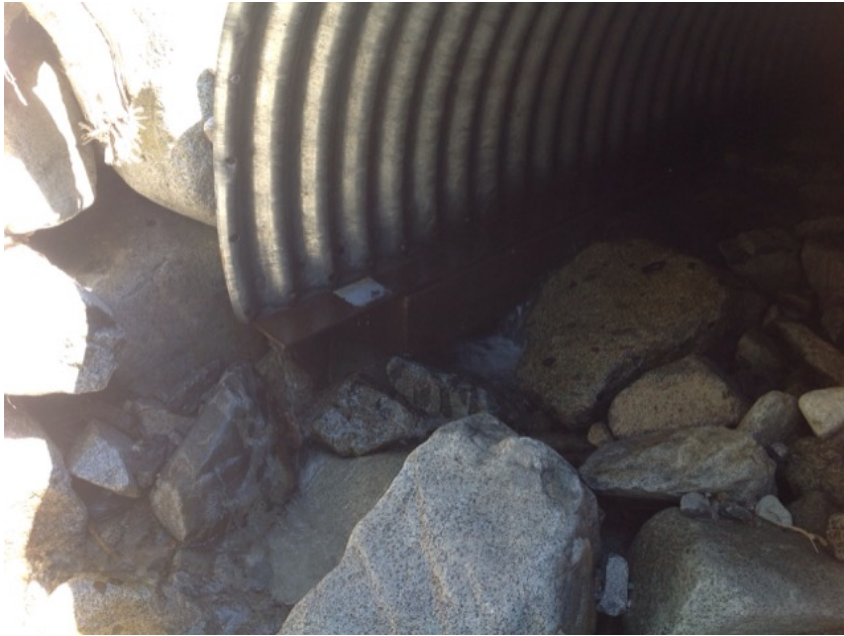
footing scour at outlet
